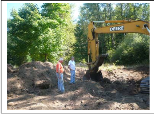
Implementation: Landowner, Eric Haws and Contractor watch as the excavation of earth begins. August 2007
